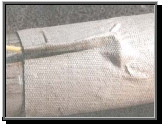
Figure 1-2. The above photo illustrates how one competitor's coating can emphasize an already weakened coating on a weld "load" point
